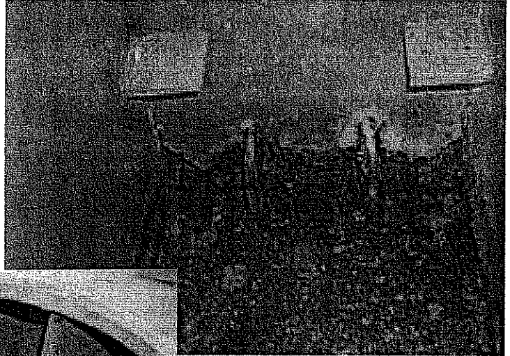
L13/U14 Corrosion @ Diaphragm
