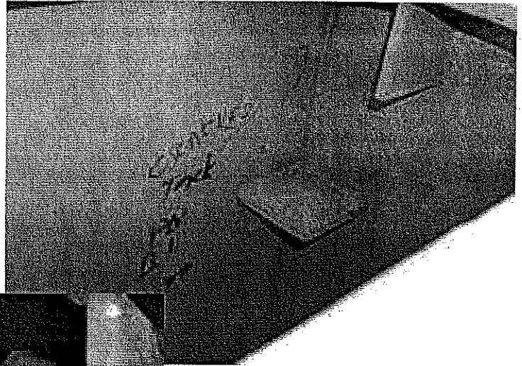
Cracked Tack Weld @ Diaphragm #3
