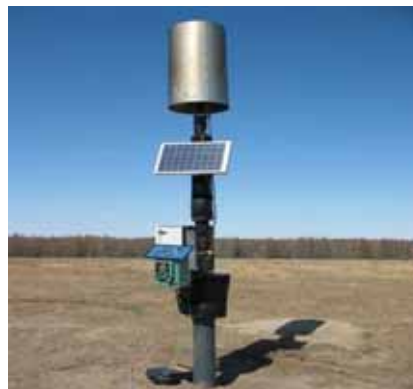
Solar flare at Kummer Landfill, Beltrami County
