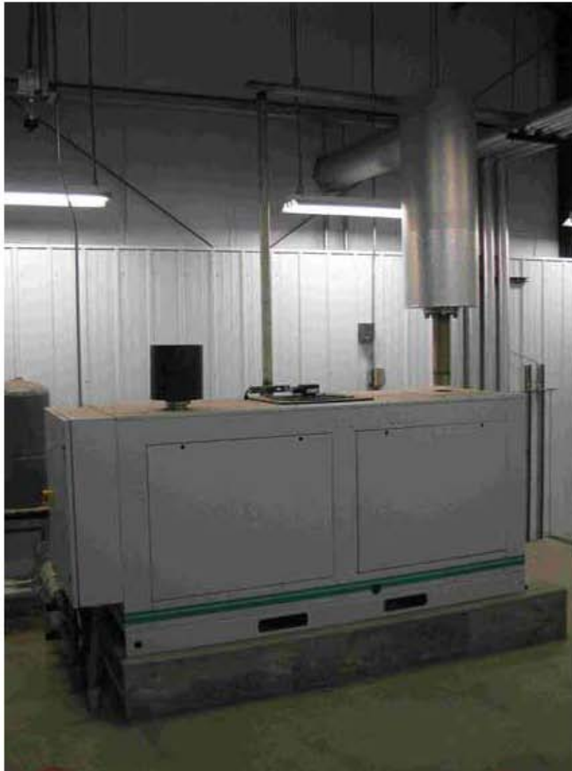
Stirling Engines for the gas-to-energy system WDE Landfill, Anoka County
