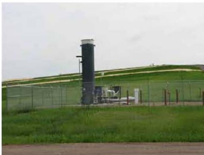
Active Gas Extraction System Flare East Bethel Landfill, Anoka County
