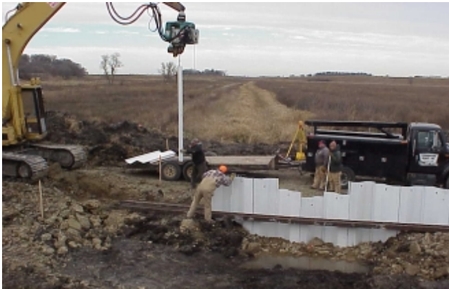
Design and engineering services are provided for wetlands restored through RIM/CREP and the Minnesota Wetland Banking Program.
