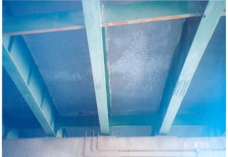
Water Saturation SB bays 15 & 16
