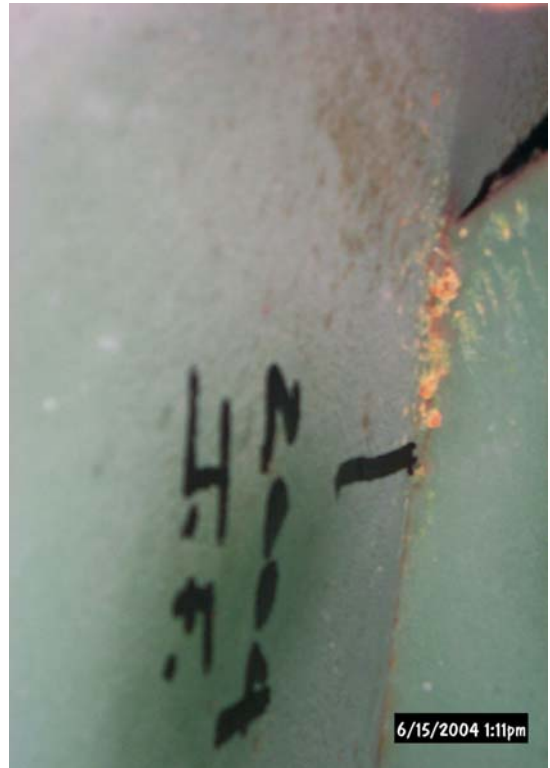
Member L14/L13' Cracked Tack Weld
