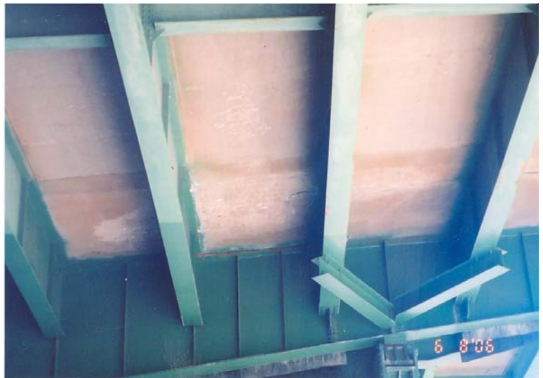
Water Saturation NBL Bays 2, 3 & 4
