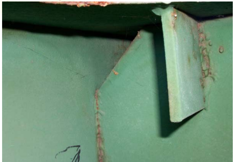
Cracked Tack Weld @ Diaphragm #2
