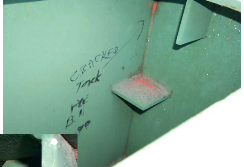
Cracked Tack Weld @ Diaphragm #3
