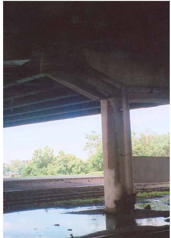
Median Drain Plugged Pier 9
