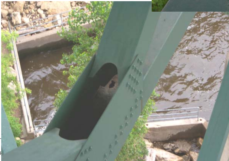
Hole in Bottom Member of Sway Bracing
