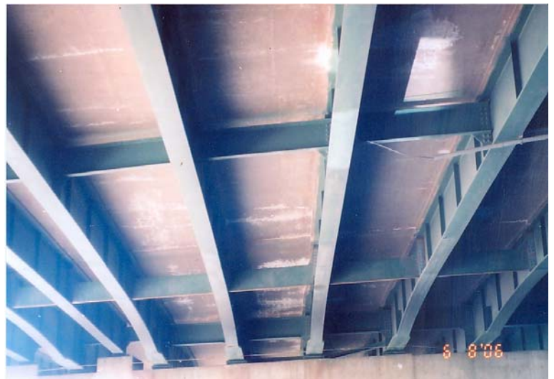
Water Saturation NB Bays 5, 6 & 7
