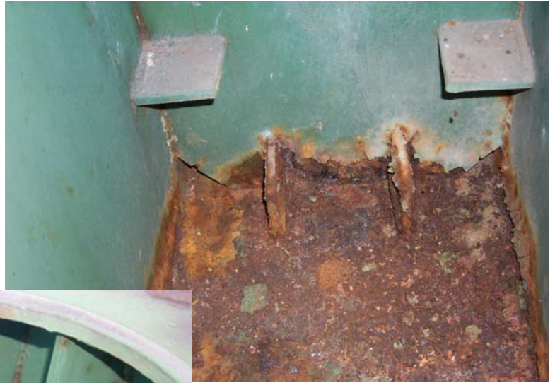
L13/U14 Corrosion @ Diaphragm
