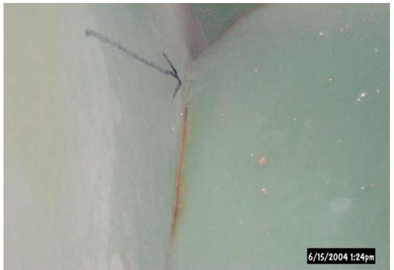
Member L13'/L12' Cracked Tack Weld
