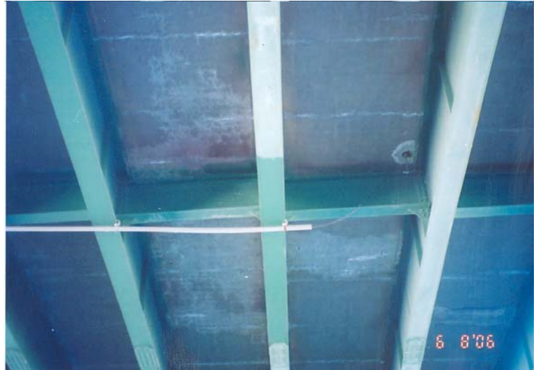
Water Saturation SBL Bays 9 & 10
