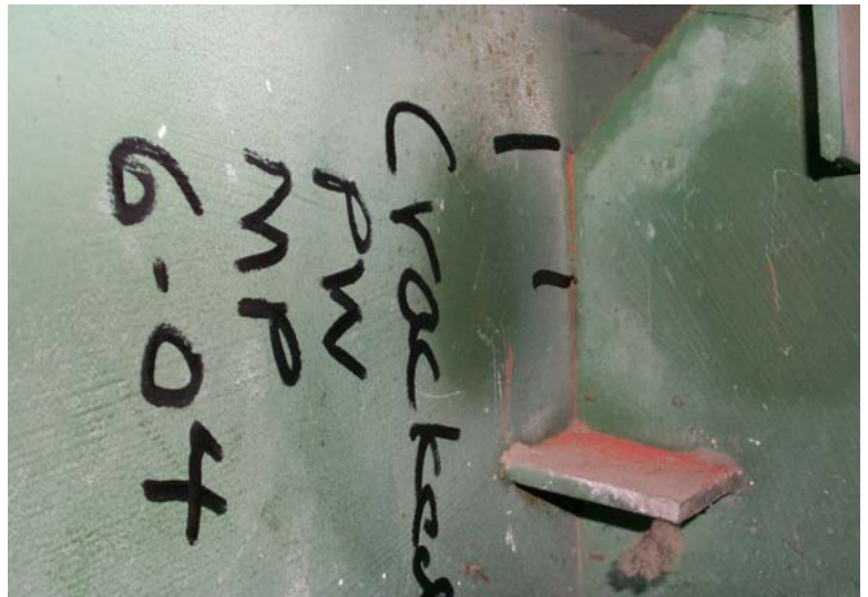
Cracked Tack Weld @ Diaphragm #2
