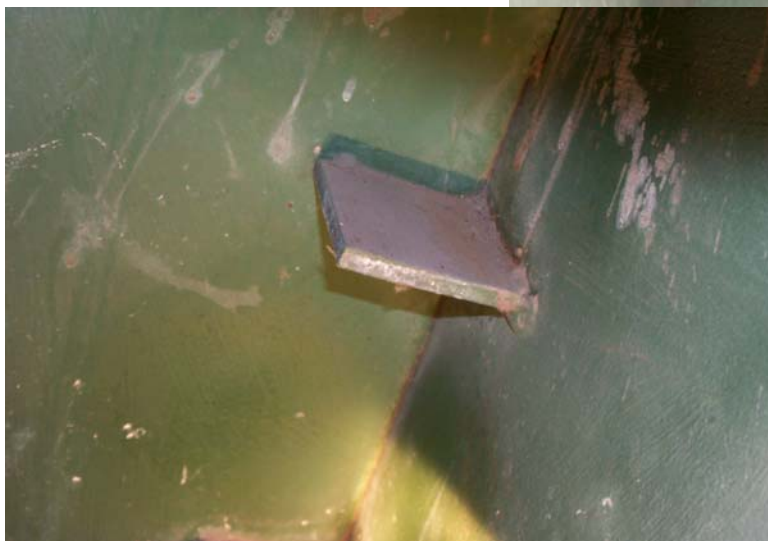
Cracked Tack Weld @ Diaphragm #1
