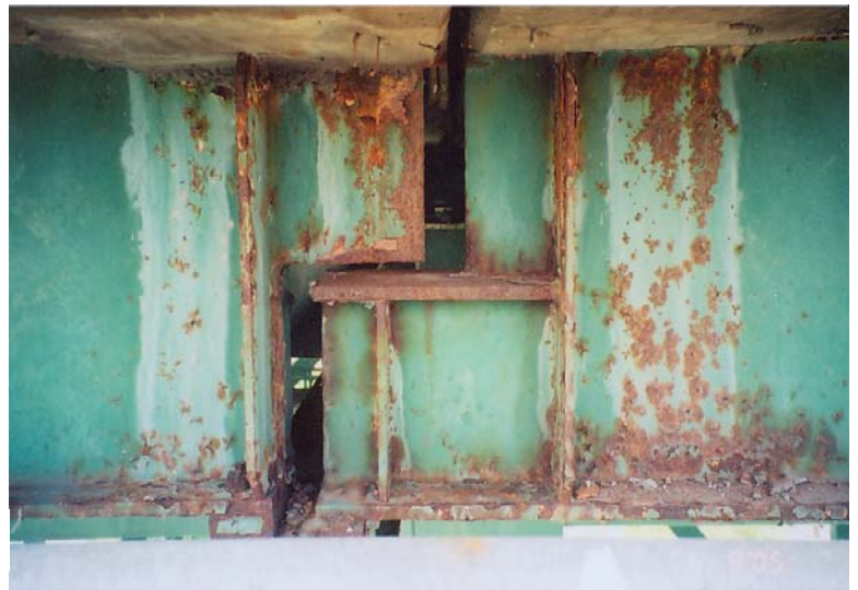
Flaking & Surface Rust Exterior East Truss
