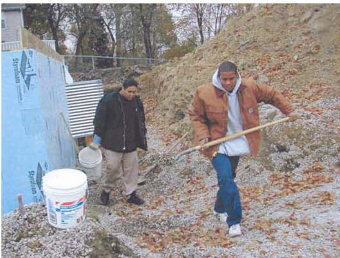
Brandon Howard and Raymond Johnson installing drain tile and egress windows on a home under construction in south Minneapolis.
