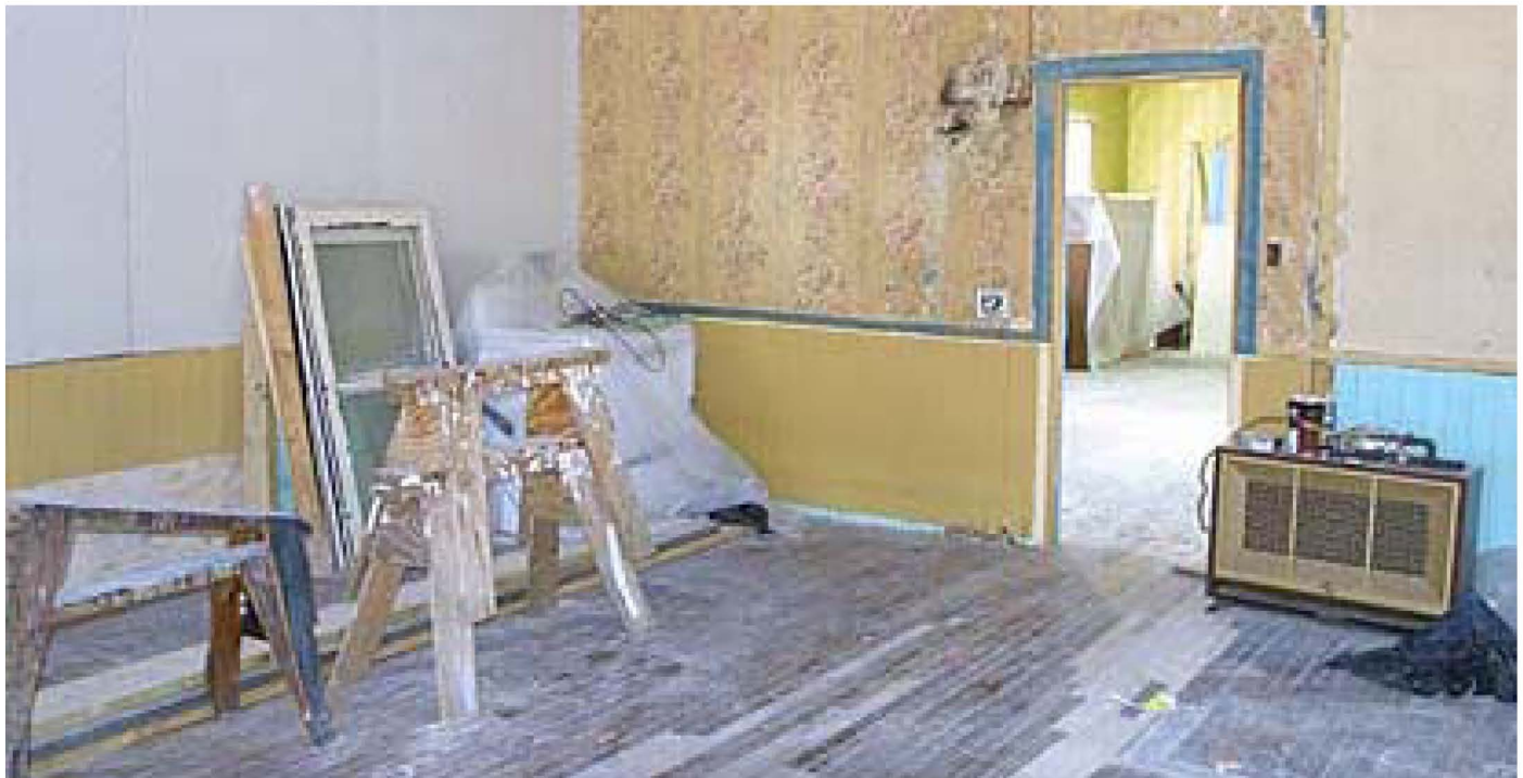
Interior renovation on the Finnish Boarding House in Chisholm is nearing completion by AEOA Youthbuilders.
