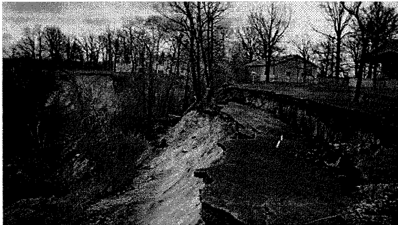
Recent Subsidence Events in Red Lake Falls, Minnesota
