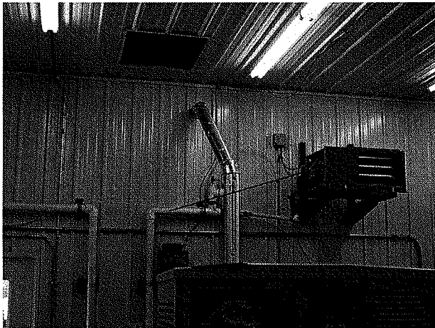
Natural Gas Heater for Testing Biogas
