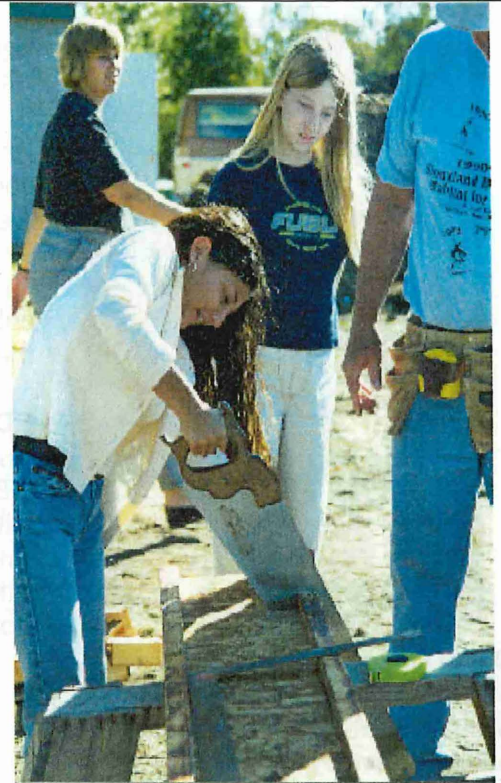
Gracie Cuellar sawing boards to be used to build walls at Demo Inc. (non-profit art museum).
