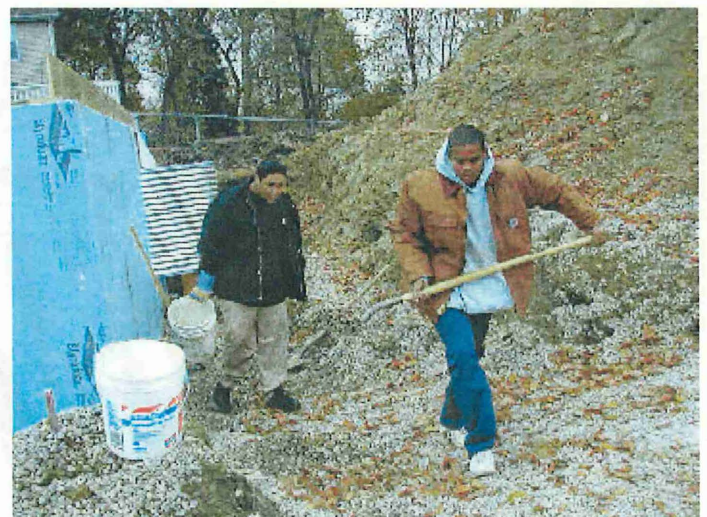
Raymond Johnson and Brandon Howard installing drain tile and egress windows on a home in south Minneapolis under construction.
