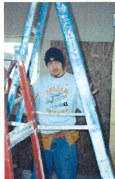
Rodney Wasche, Perham Youthbuilder, paints ceilings and interior walls of newly constructed house.
