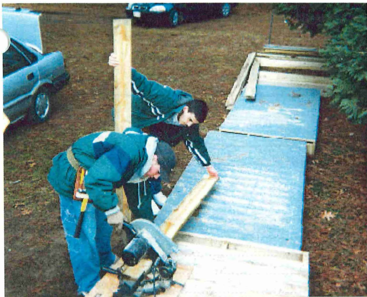
Brett Gremminger and Jon Wilson saw boards while building a wheelchair ramp for an elderly homeowner.
