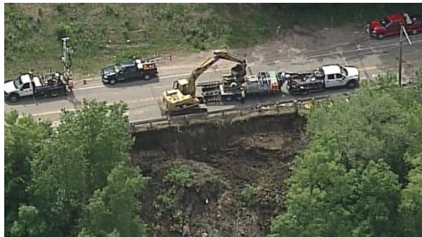
Figure 3. Highway 13, Great Rivers Trail failure in Mendota Heights. Photo from http://www.myfoxtwincities.com/story/25740202/mudslide-closes-highway-13-in-mendota .
