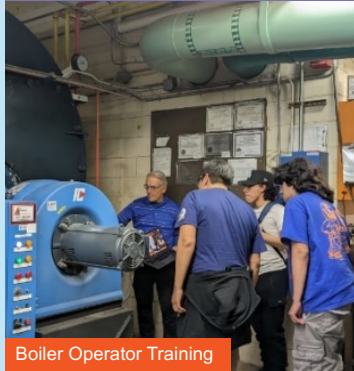
Boiler Operator Training
