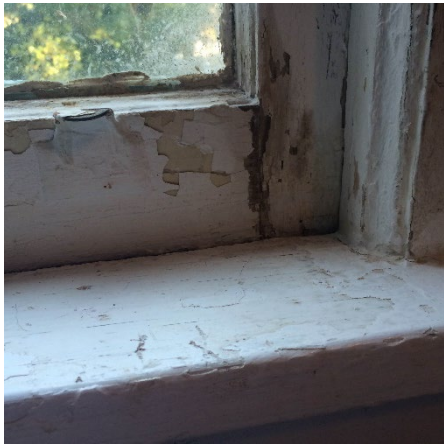
Chipped or peeling lead paint
