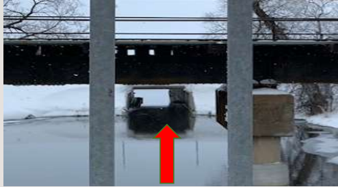
GENEVA - LE HOMME DIEU CHANNEL (UNDER HWY. 29) APPROX. DIMENSIONS 8' 8" WIDE X 4' HIGH
