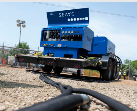
Using innovative ZEVAC vacuum pump technology to avoid gas venting when pipelines are taken in and out of service
