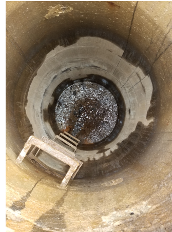
Infiltration at Manhole Structures
