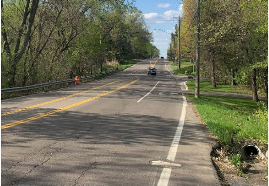
No facilities or shoulder for pedestrians and cyclists along a Tier 1 corridor or at crossing to three schools
