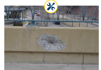
Concrete spalling on barrier
