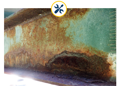
Structural member coating and section loss
