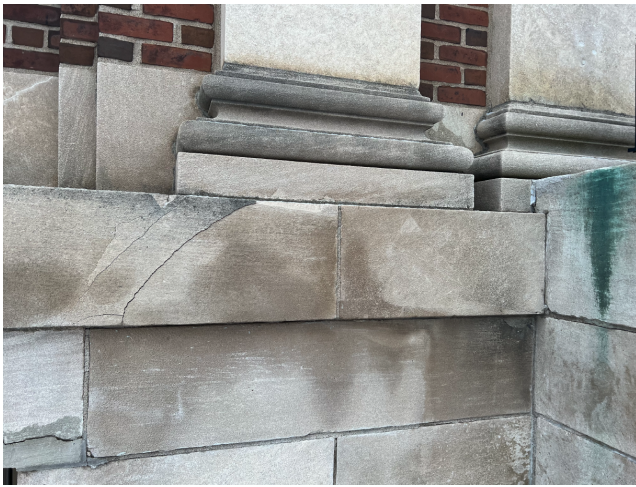
Stained and damaged stone on exterior wall.
