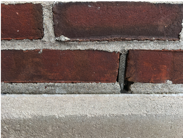
Damaged brick mortar joint on exterior wall
