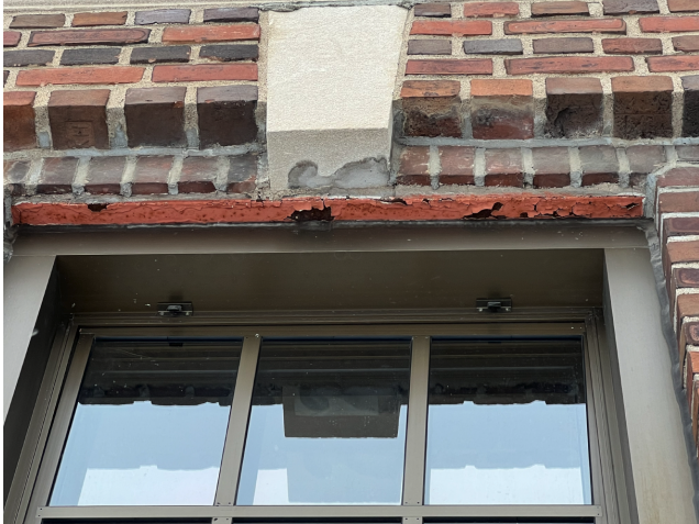
Rusted steel lintels and damaged sealant on exterior wall
