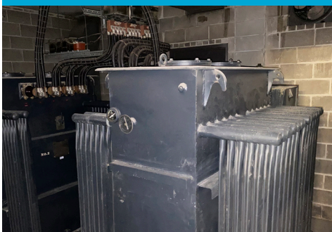
Top: ice chiller plant, middle: air handling unit, bottom: electric transformer.
