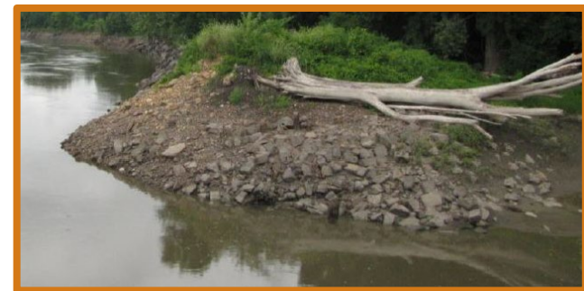
Erosion of the riverbank along the Minnesota River in the project area
