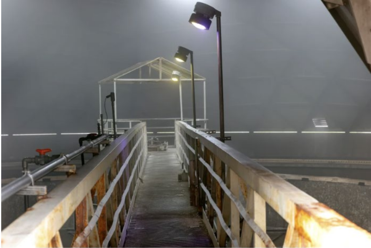
A walkway leads to the center of the failed secondary clarifier at the Western Lake Superior Sanitary District. Because of structural damage, only one person can enter the structure at a time. Repairs may have to be made from above. Steve Kuchera / Duluth News Tribune
