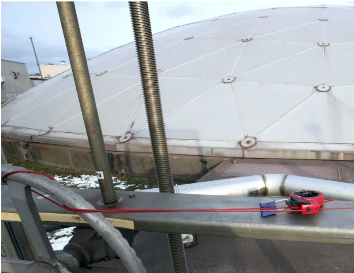
A cable and lock prevents anyone accidentally turning on the broken secondary clarifier, background, at the Western Lake Superior Sanitary District. Steve Kuchera / Duluth News Tribune
