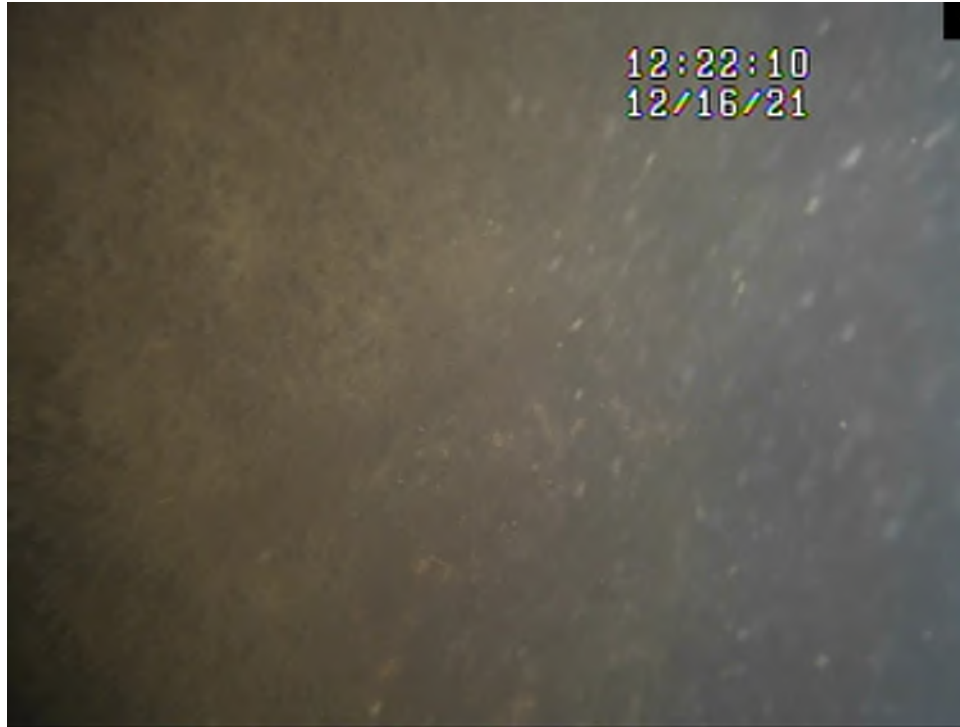
Figure 2 - Concrete Sill: Marine Growth
