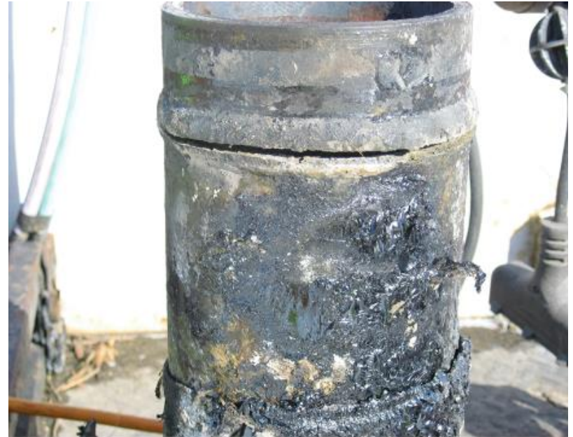
UM-Crookston Ruptured Natural Gas Main
