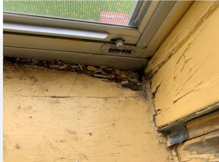
Deteriorating Windows in Living Units
