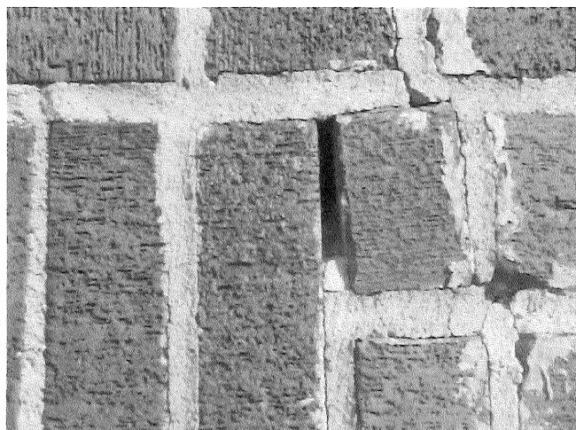
Building deterioration due to age.
