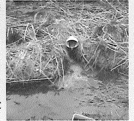
Drain pipe emptying into ditch
