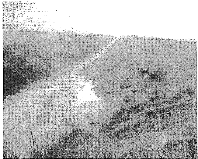
The photo above shows sloughing of the ditch bank in JD #9.
