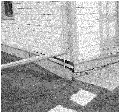
Damaged Ice House Foundation
