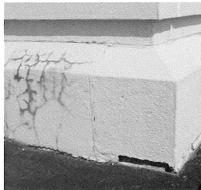
Damaged Lighthouse Foundation
