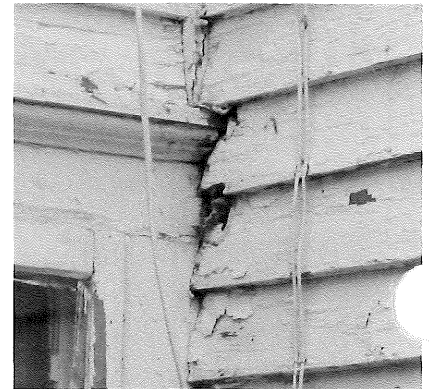
Rotted Store Siding
