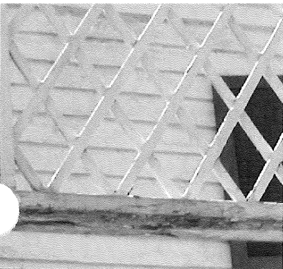
Rotted House Railing
