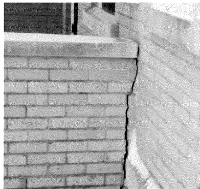
Cracked Dwelling #3 Porch
