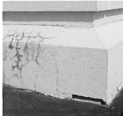
Damaged Lighthouse Foundation
