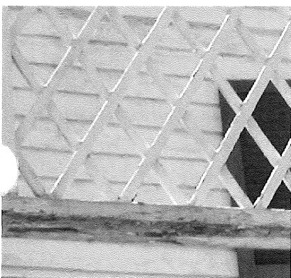
Rotted House Railing
