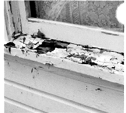
Rotted Store Window Sill
