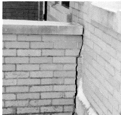
Cracked Dwelling #3 Porch
