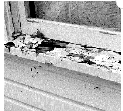
Rotted Store Window Sill
