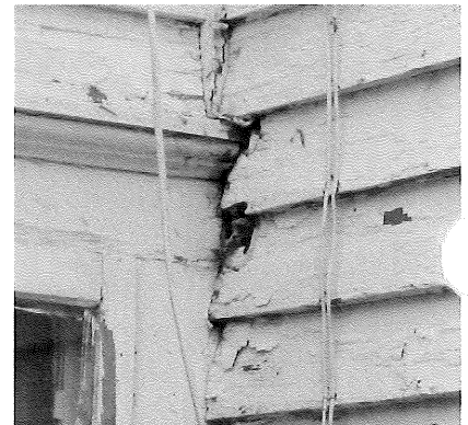
Rotted Store Siding
