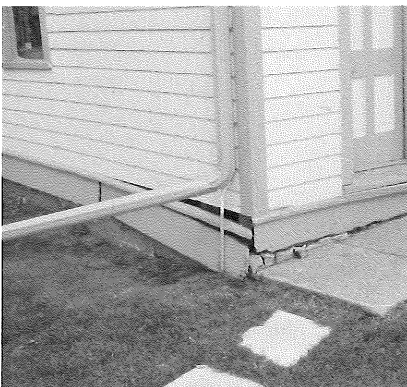
Damaged Ice House Foundation
